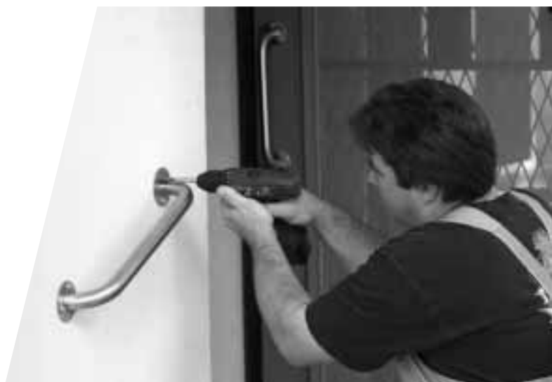
Installing a handrail for home care residents, as part of the home and community care program.
