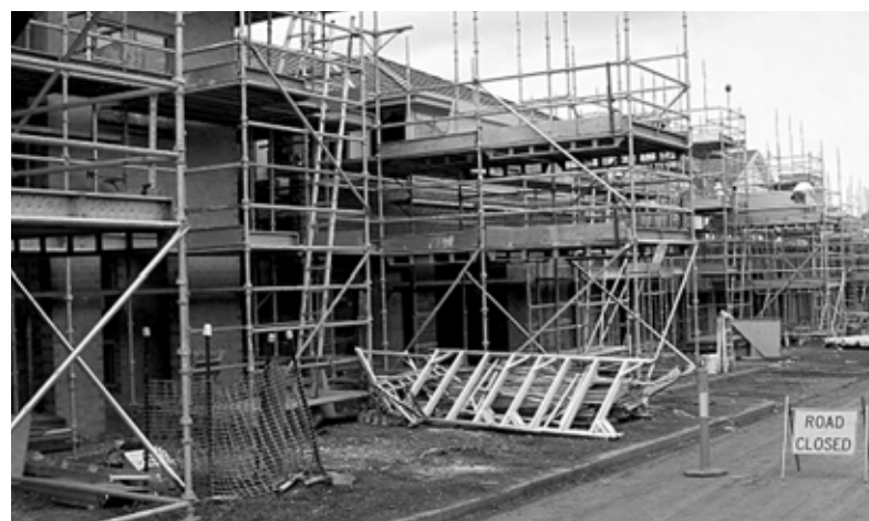
Houses under construction in the Commonwealth Games Athletes' Village. (Photo courtesy of Major Projects Victoria.)
