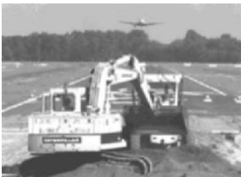
Extension of runway at Shepparton Airport located in the North East Region of Victoria, partly funded by the Regional Infrastructure Development Fund.
