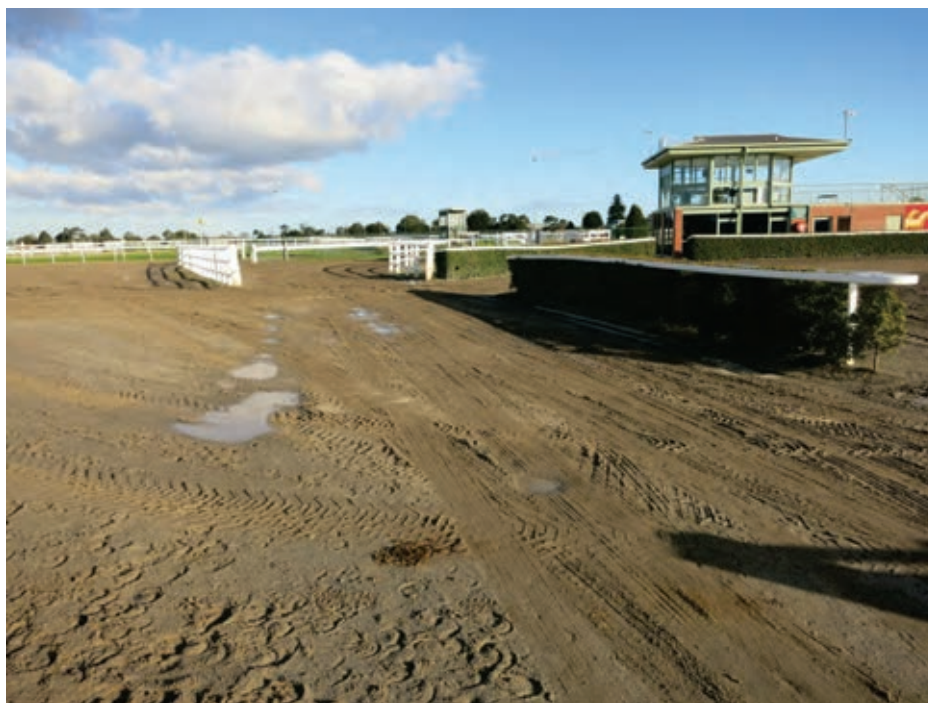
Public reserve—condition of the track from Glen Eira Road tunnel to car park.
