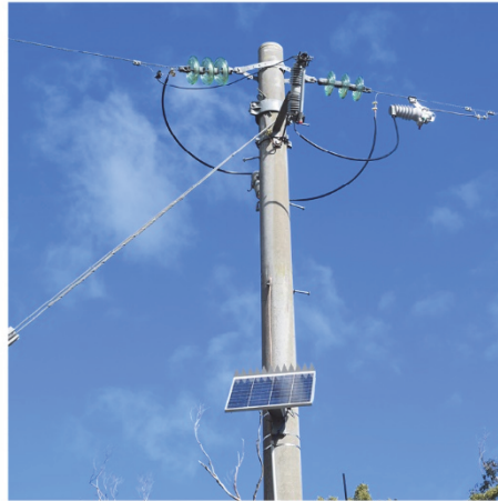
12.7kV Single-wire earth return powerlines. These single-wire powerlines run across regional Victoria and were installed when the network was first built. They are cheaper to construct and maintain than multi-wire powerlines.
