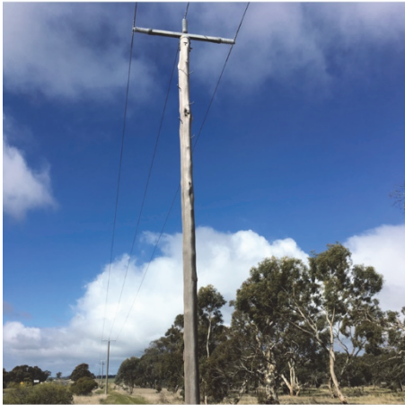
22kV Three-wire powerlines.
